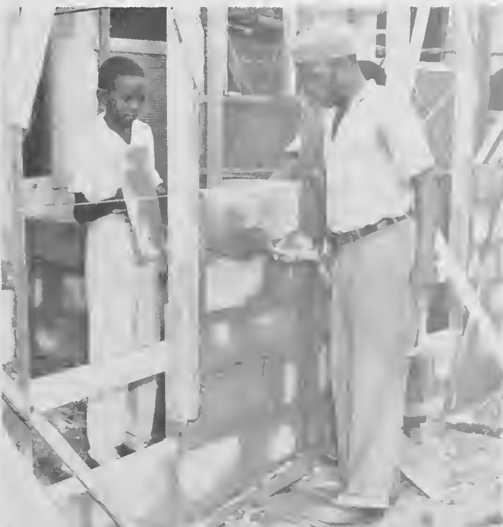
CONCRETE BLOCKS were used to add kitchens to the two apartments in the building. Thanks to plenty of hard work, the building has been finished, and put to excellent use by people who needed a roof and a home.
